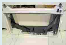
106Gal. Gas Tank under floor
